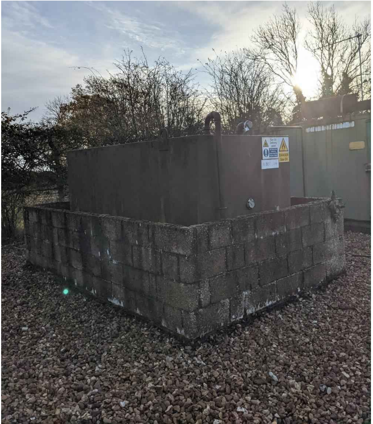
Photo 1: Waterbeach WRC fuel tank
